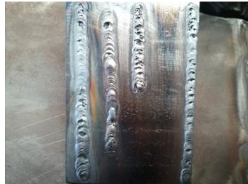
Weld is porous
